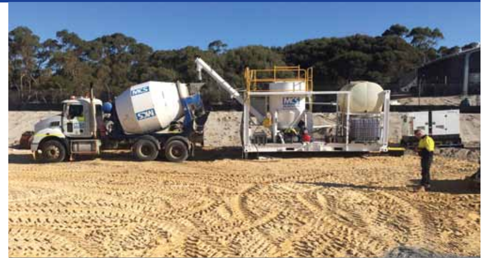
Above: Construction work has commenced on the eco-resort at Pinky's, Rottnest Island.
